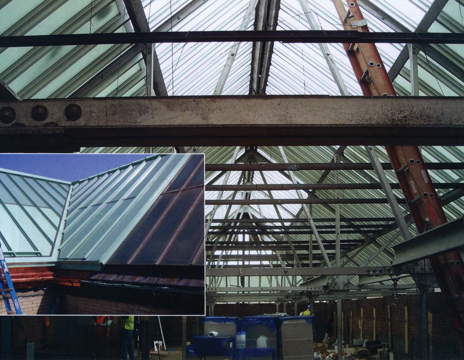
The Corcoran Gallery's original wired glass skylight was replaced with laminated insulating glass units.
